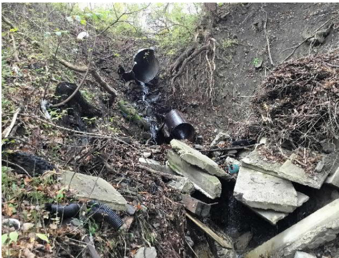
Carmichael Road over Tributary to Huntington Creek. Structure outlet, showing severe erosion and collapse of outlet section.
