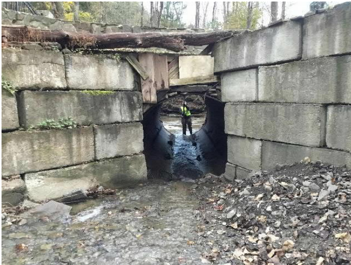
Private (Winery) Driveway off Allen Glen Road over Huntington Creek. Structure inlet. Note plywood in place of headwall and misaligned wingwalls.
