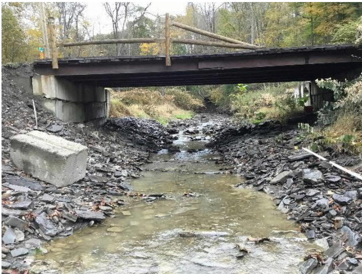
Private Driveway off Dean Street over Huntington Creek (downstream). Structure inlet. Note sagging abutment and displaced concrete waste block on left bank.
