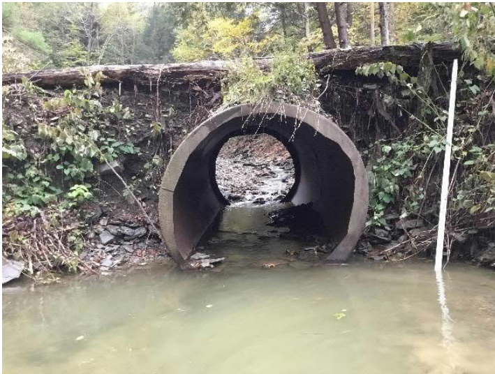
Private Driveway off Dean Street over Huntington Creek (upstream). Crossing structure outlet. Note erosion of road embankment on either side of structure.
