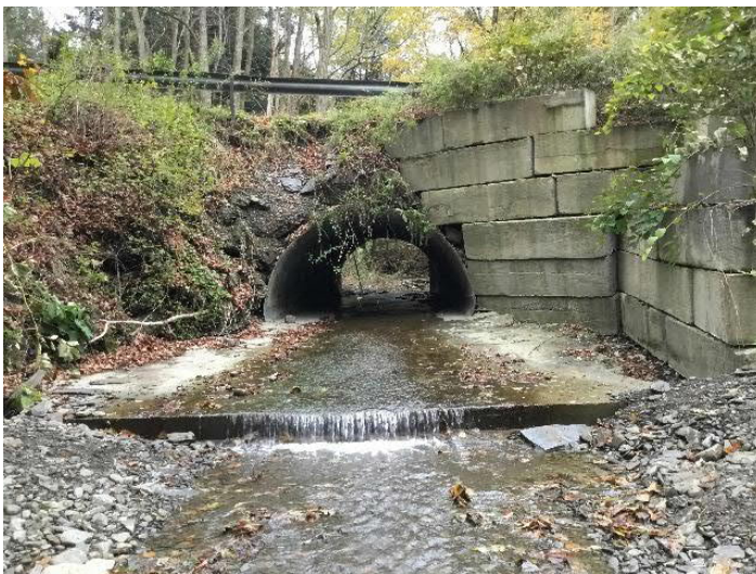
Allen Glen Road over Huntington Creek. Structure outlet. Note unstable wingwall and concrete-lined streambed, eroding road embankment, and outlet drop.
