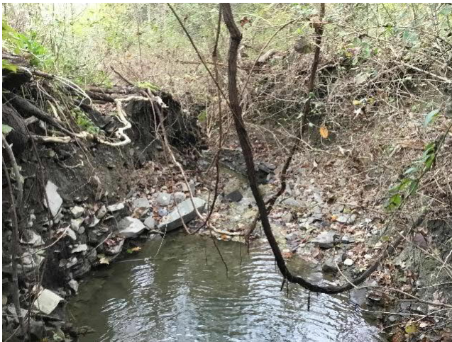
Private Driveway/Access Road off Carmichael Road over Tributary to Huntington Creek. Severely incised/eroded channel downstream of structure.
