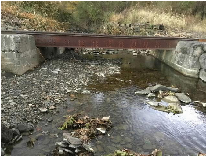
Outlet of Owego & Hartford Railroad bridge over Huntington Creek. Note low bridge clearance, constriction of stream by bridge abutments, and timber retaining wall lining upstream channel.
