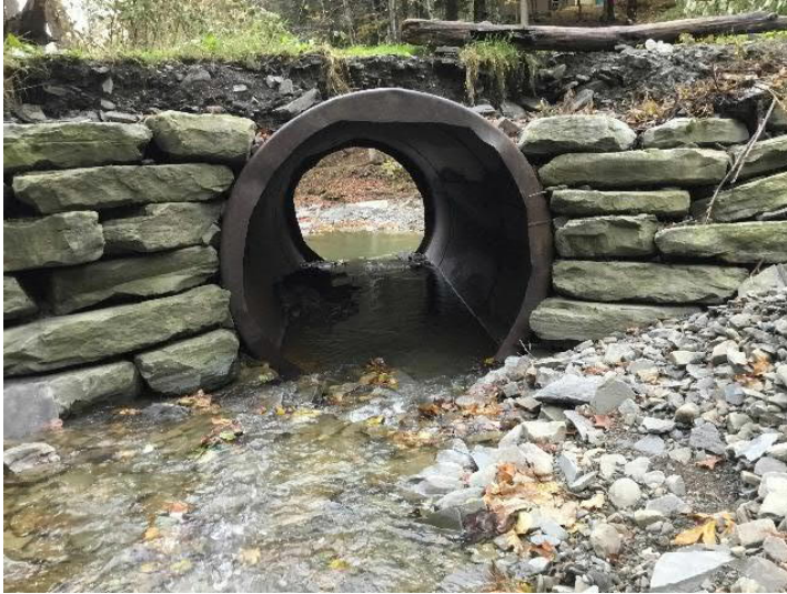
Private Driveway off Dean Street over Huntington Creek (upstream). Close-up photograph of structure inlet. Note inadequate fill/cover material above culvert, erosion of road along top of structure, and sediment deposition on river right.
