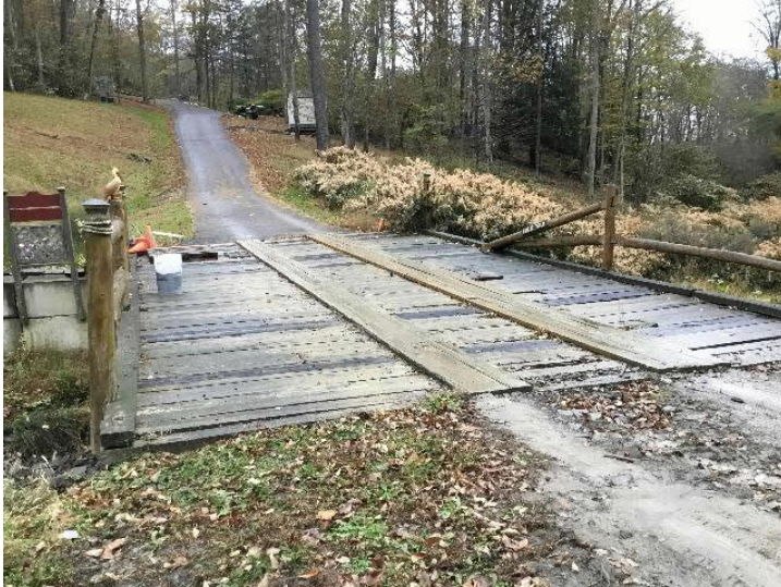
Private Driveway off Dean Street over Huntington Creek (downstream). Photograph of bridge deck. Note planks placed lengthwise on bridge deck to support vehicle traffic.
