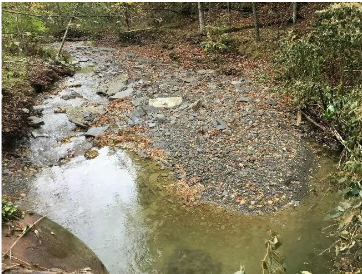
Private Driveway off Dean Street over Huntington Creek (upstream). Streambank erosion on river left and deposition on river right, downstream of crossing structure.
