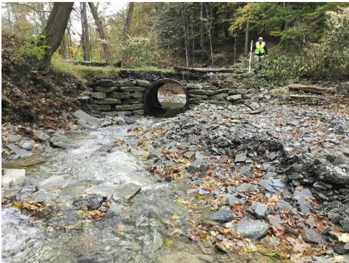
Private Driveway off Dean Street over Huntington Creek (upstream). Structure inlet. Note erosion of road along top of structure, and sediment deposition on river right.
