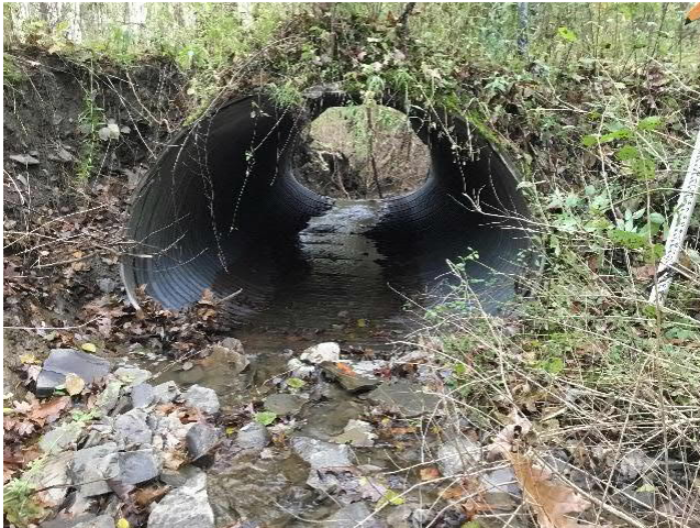
Private Driveway/Access Road off Carmichael Road over Tributary to Huntington Creek. Structure inlet. Note erosion on left side of structure.
