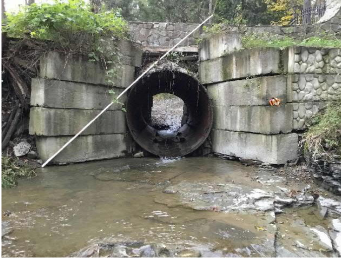
Private (Winery) Driveway off Allen Glen Road over Huntington Creek. Structure outlet. Note debris and plywood in place of headwall and severely misaligned wingwalls.
