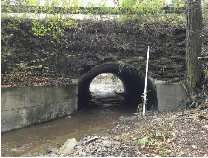
Allen Glen Road over Huntington Creek. Structure inlet. Note missing headwall exposing embankment formed of stacked bags of grout.
