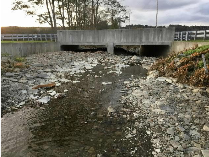
Inlet of Sheldon Guile Boulevard crossing over Huntington Creek. Note sediment nearly filling culvert structures.
