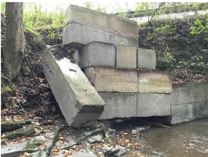
Allen Glen Road over Huntington Creek. Severely unstable wingwall upstream of structure inlet.
