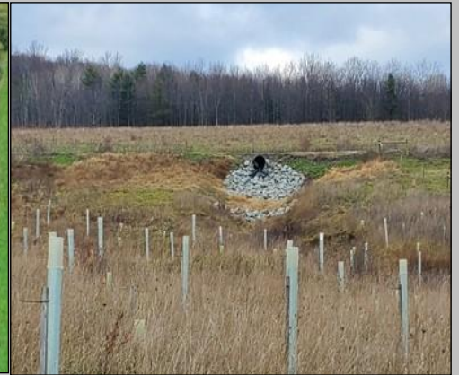
Grade control structures at a road culvert outlet into field in Chemung County (Town of Chemung)
